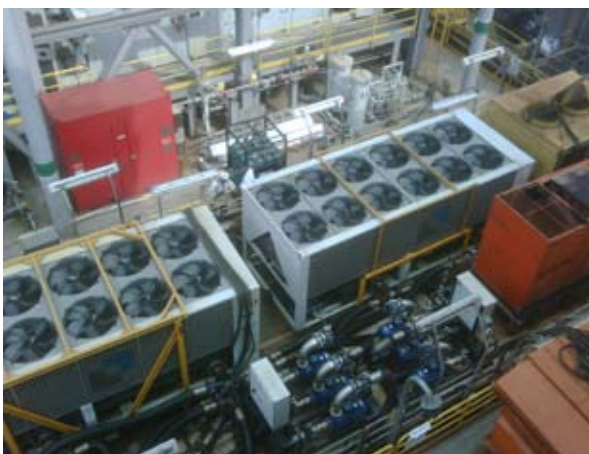
Cool Energy's 4.5mW package operating in 40°C ambients
