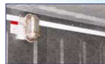
Internal lighting safety lights and lamp with sensor
