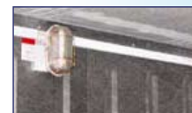
Internal lighting safety lights and lamp with sensor
