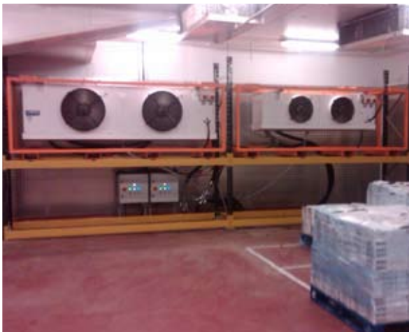
2 x 50kW low noise fan coils in situ
