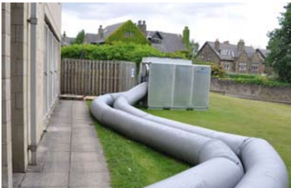
Externally sited temporary solution
