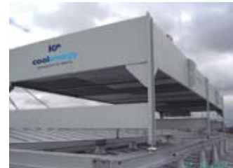
HVAC or Process Equipment
