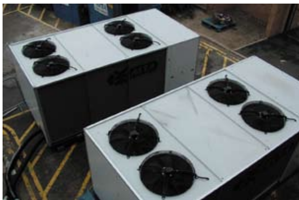
Freeze Damage - Chiller Rental
