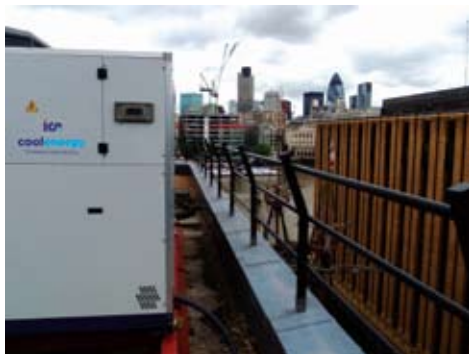
Temporary Cooling - Fast.
