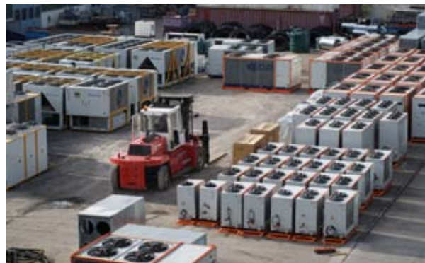
Cool Energy Depot in Hagen, Germany.
