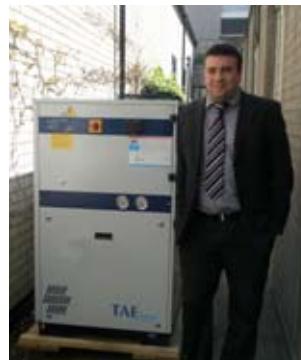
Rental Engineer, Lee Chard on site with the chiller system
