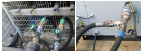
Connections to the Chiller and Flexible hose connections
