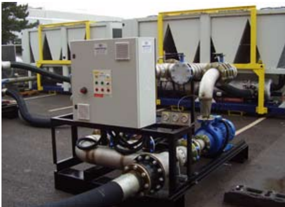
The 650kW low noise chillers on site
