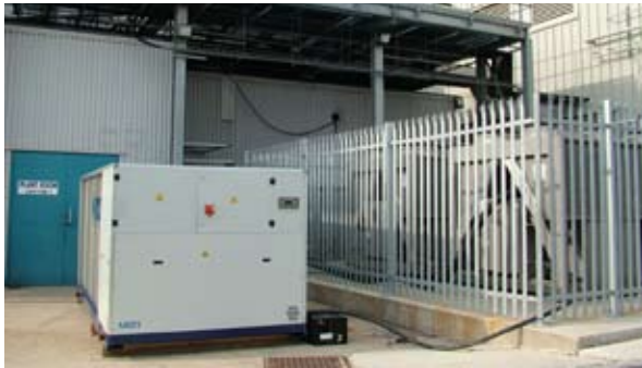
Cool Energy 250kW rental chiller supplied during the retrofit of an R22 Chiller.
