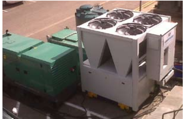
Temporary power package and fuel management
