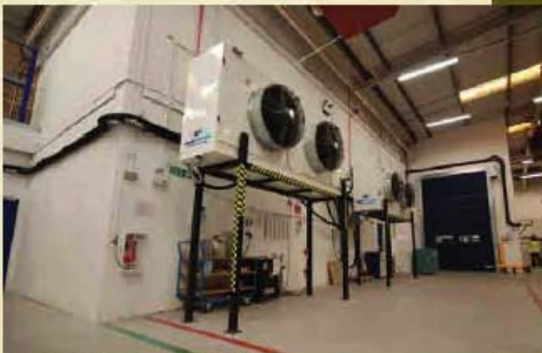
Regional distribution centre cooling project
