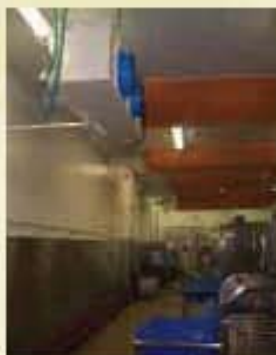
Ceiling mounted low temp coil
